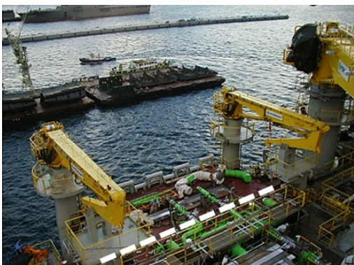
Figure 14: Leak point monitoring of offloading nozzles at a FPSO LPG offloading area
