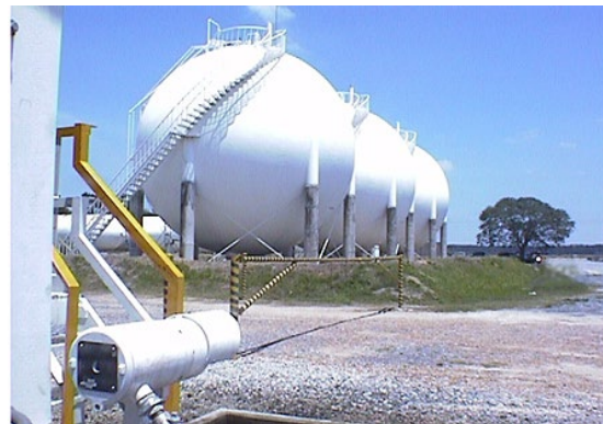
Figure 16: OPGD monitoring at boundary of LPG storage tank farm
