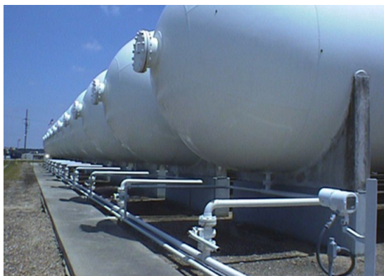
Figure 15: Leak point monitoring of a row of valves
